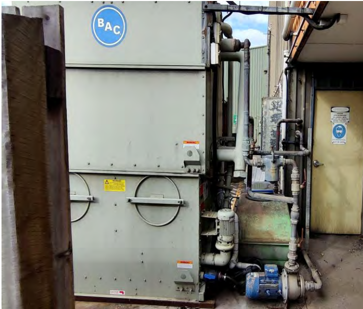
Original BAC closed-circuit cooling tower — removed
