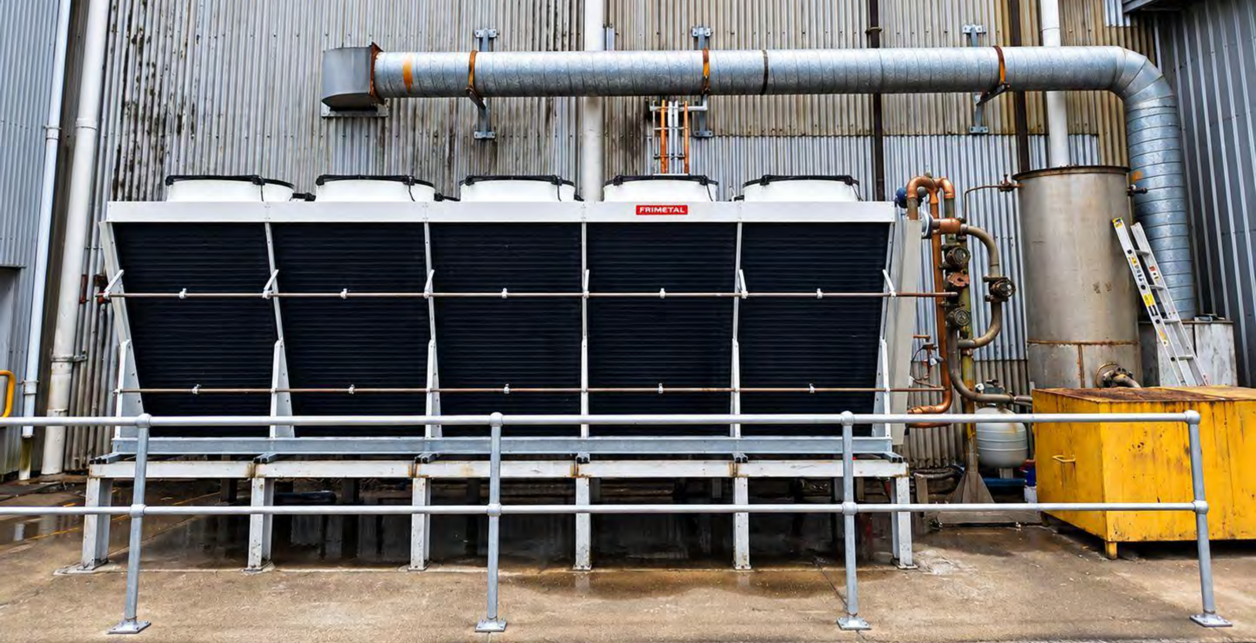
10 Fan "V" shape Cooler QLD 1500 kW Melter.
