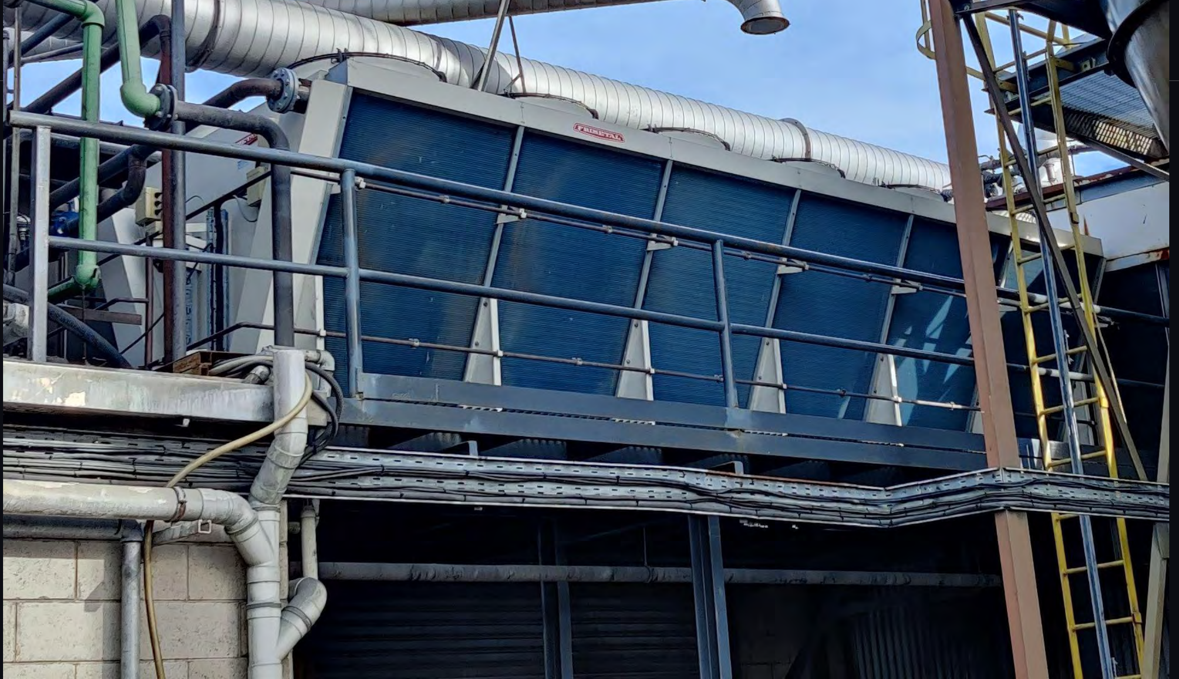
12 Fan “V” shape Cooler Christchurch NZ cooling multiple Induction furnaces totalling more than 2100 kW
