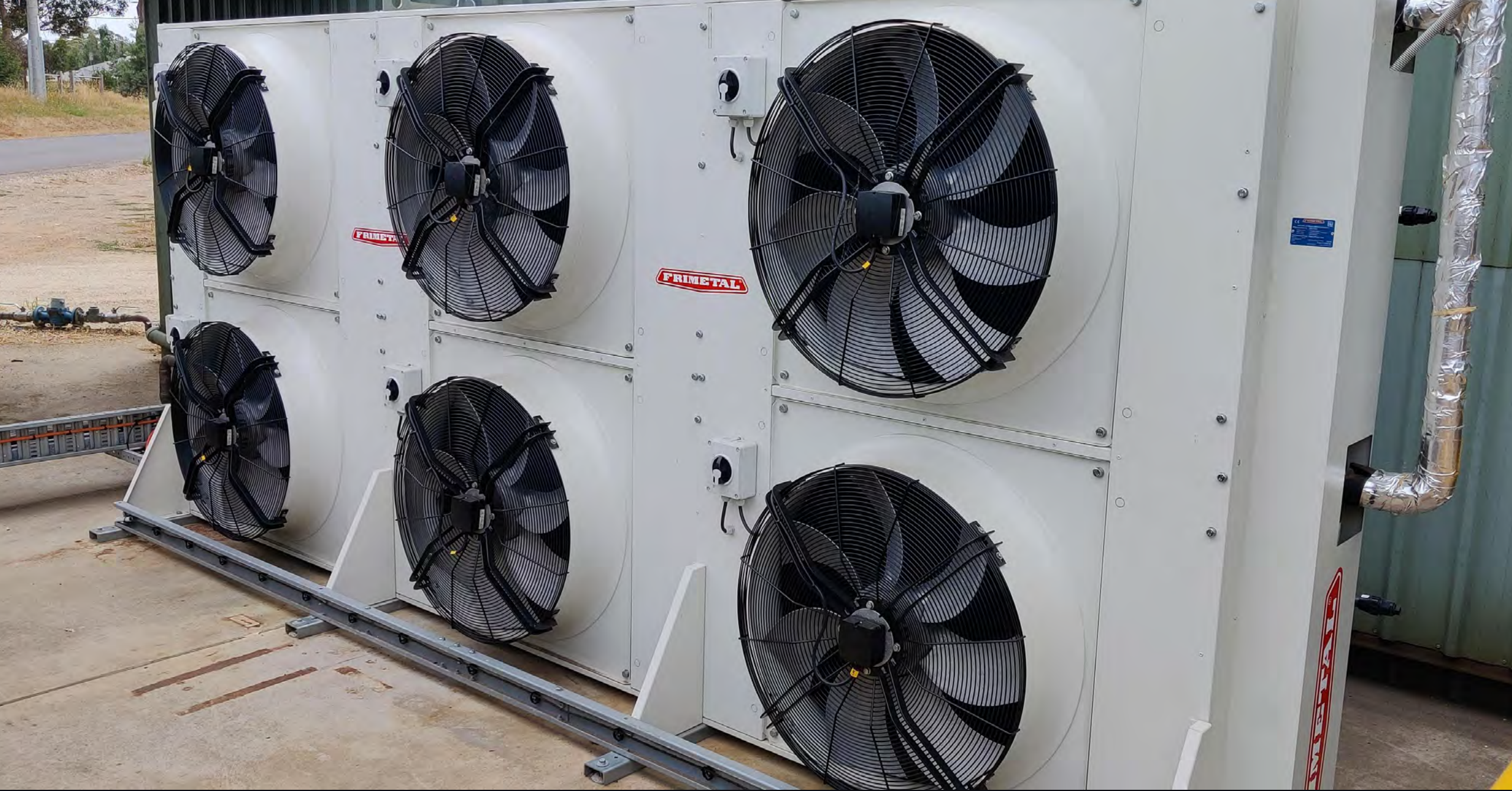
Compact space saving Six Fan flat vertical Cooler – Castlemaine Vic.
