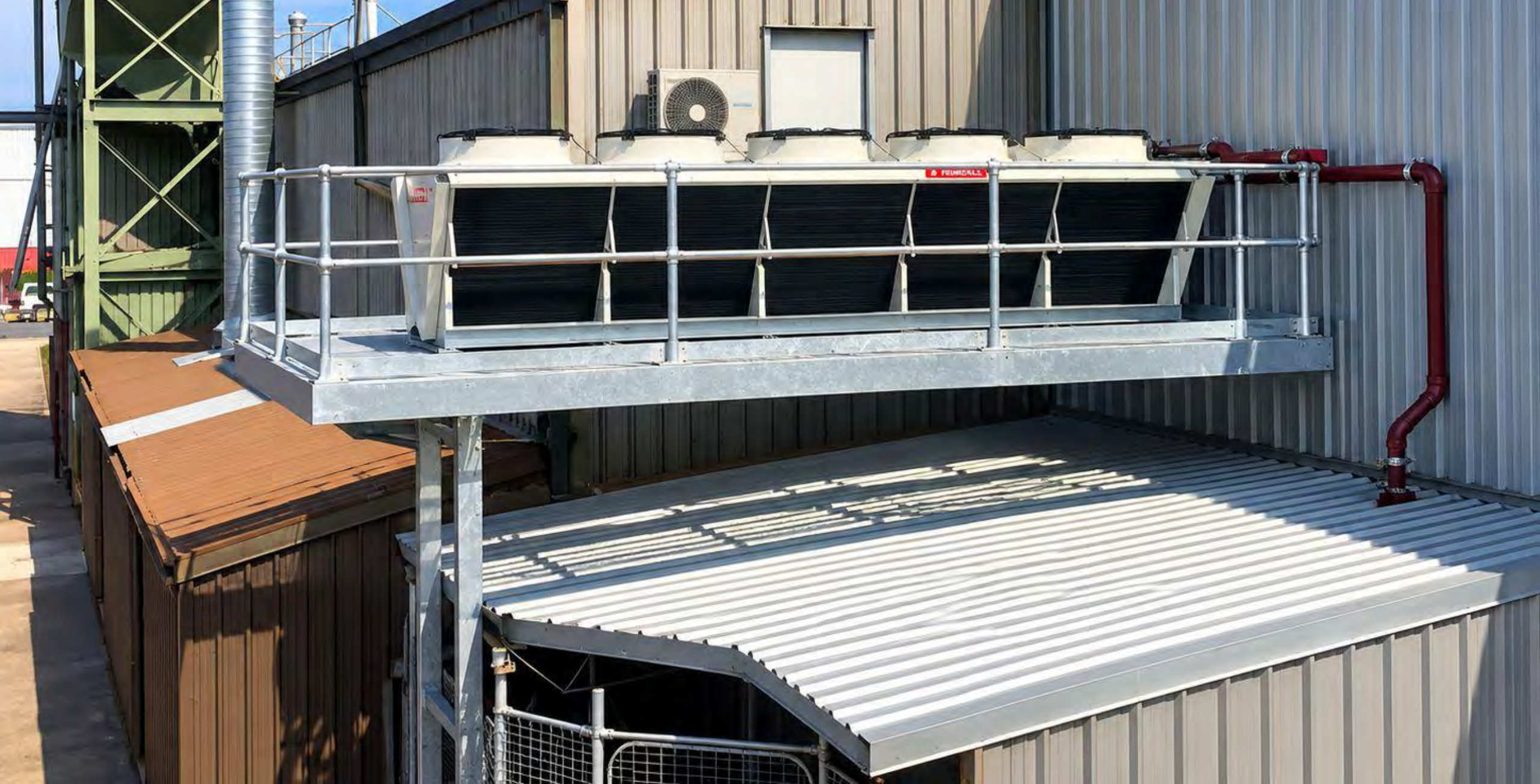
Five Fan “V” Shape Cooler - Brisbane. This customer has ordered a second 5 fan cooler to suit his expanding melt shop
