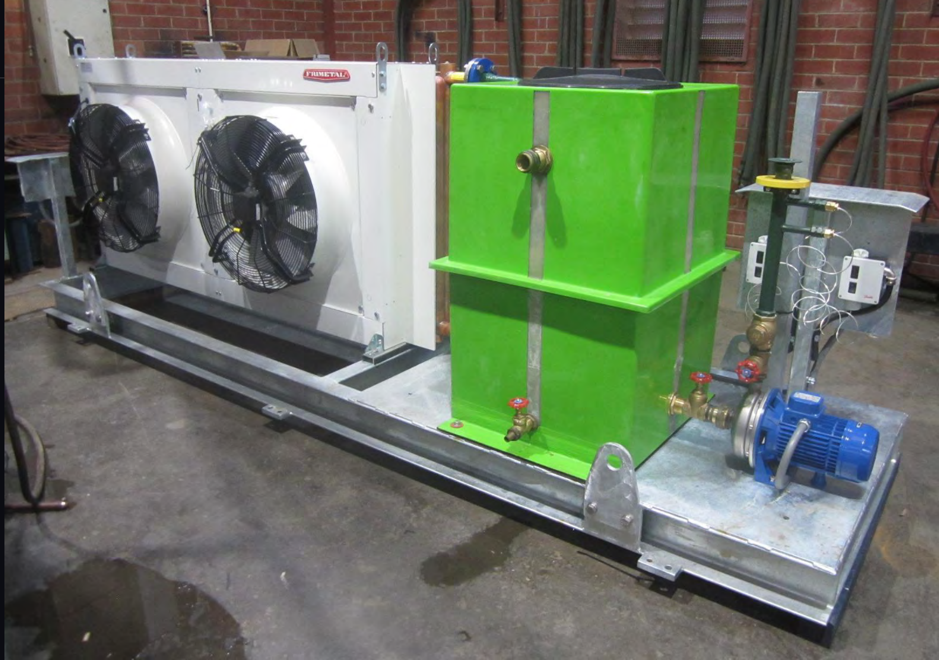
Two Fan Cooler water module for a Victorian Mine site
